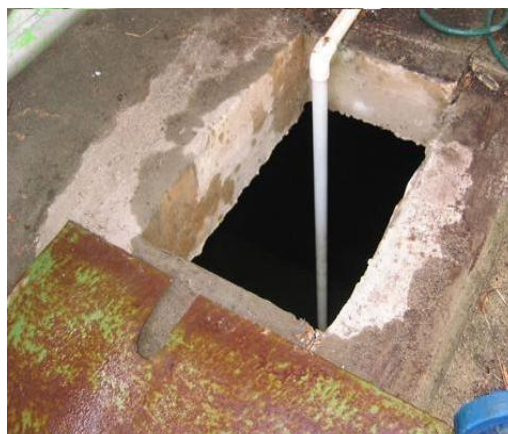
(F-4.4T-RO U/G sump)
