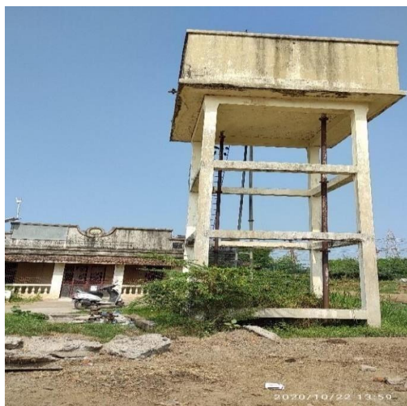
(F-4.4A-Overhead Water tank)
