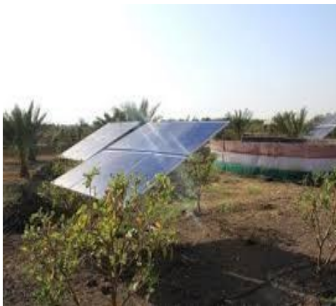
(F-4.4S-Solar Panel System)
